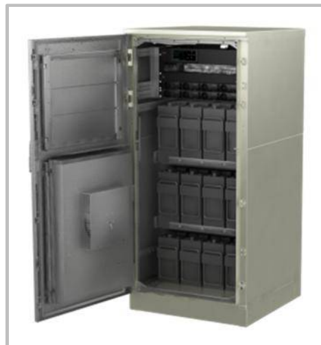
FLATPACK2 SYSTEM IN TYPE3 OUTDOOR CABINET
